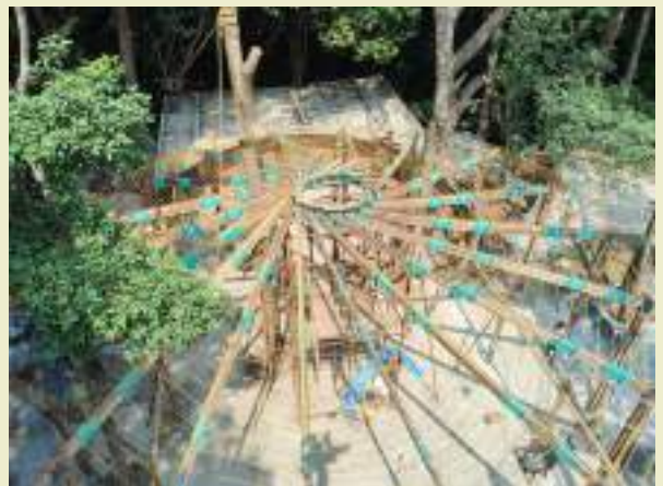
Aerial view of the conference hall's reciprocal roof structure at Devadhare. ©Patrick Gowda AK.
