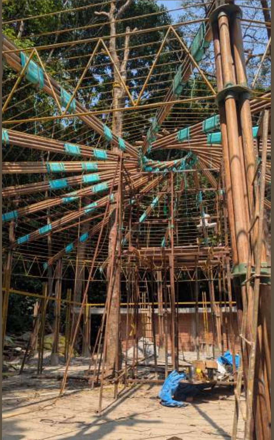
Interior view of the conference hall, highlighting the reciprocal roof at Devadhare. ©Patrick Gowda AK.
