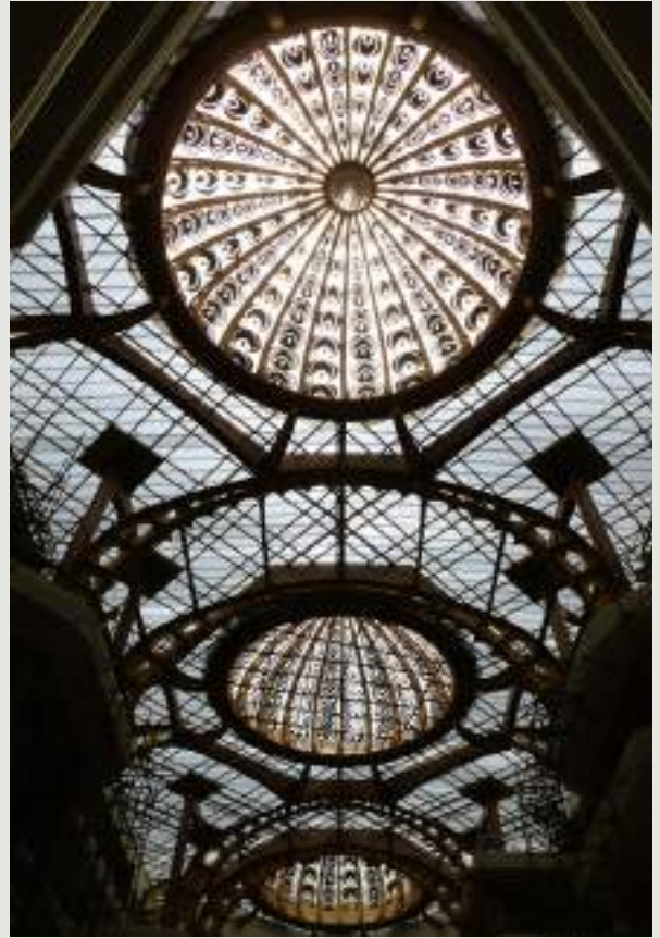
At The Celebration Mall, steel-framed Mewari domes reinterpret tradition while patterned fiberglass filter daylight deep inside making roofs both symbolic and sustainable | Courtesy: Abhikram
