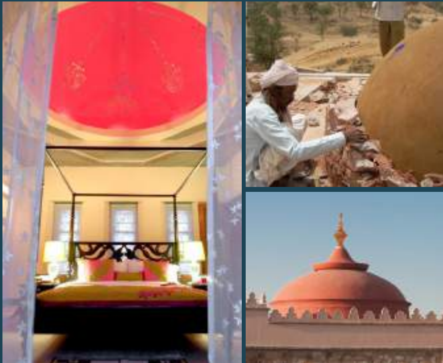
An artisan shaping the mud-based formwork, reviving time-honoured techniques of domed construction at Tree of Life Resort | Courtesy: Abhikram & Tree of Life
